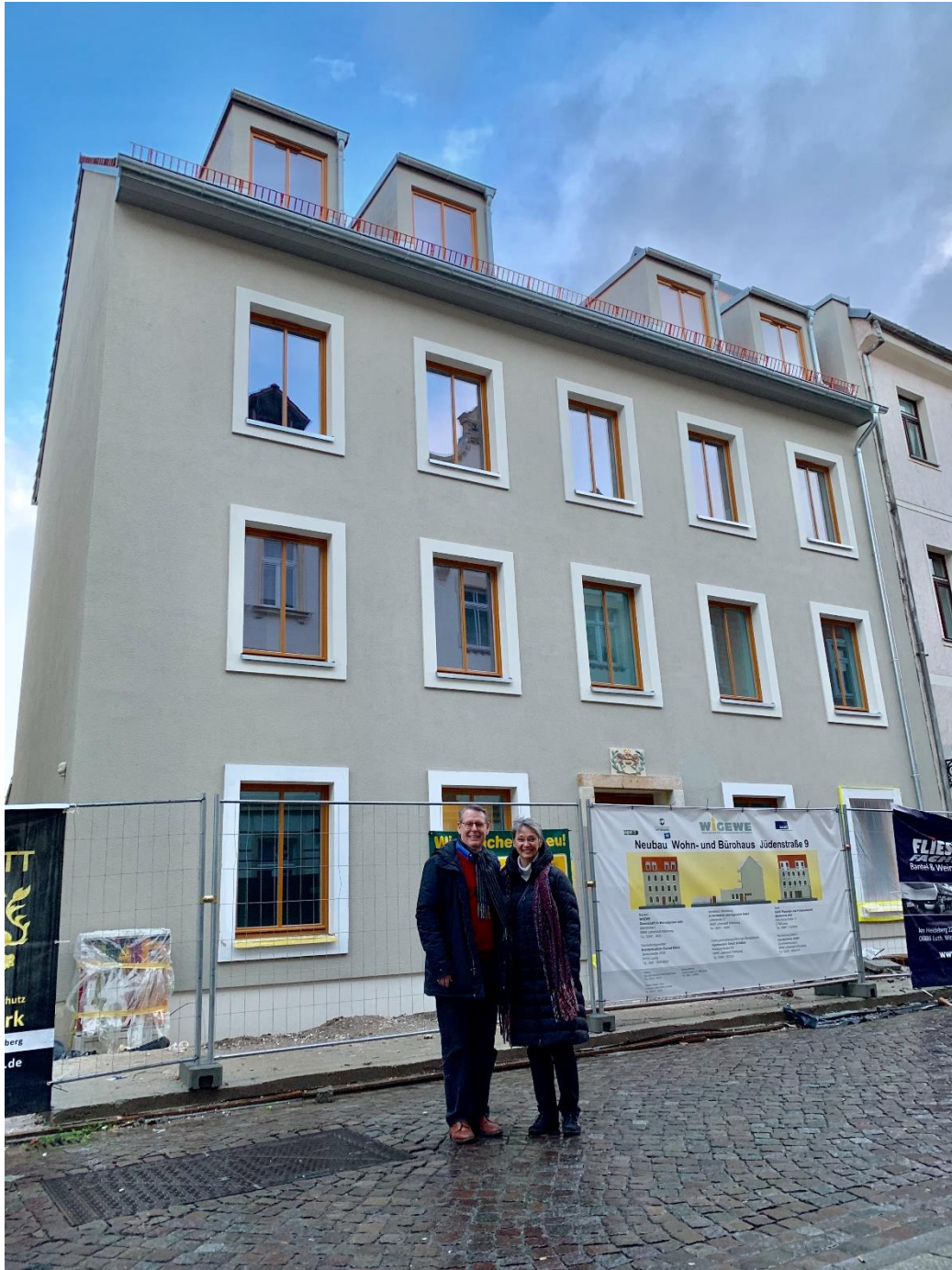
Offices for the Wittenberg Centers of the ELCA and the Lutheran World Federation are nearing completion.
